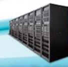
Complete Rack Solutions
